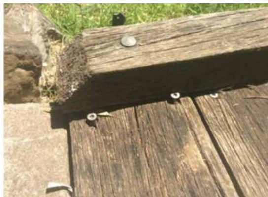
Defect – Seasonal movement – bolt lift
