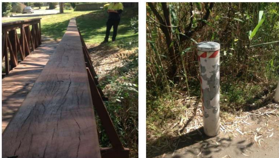
Defect – Protective Coating Failure
