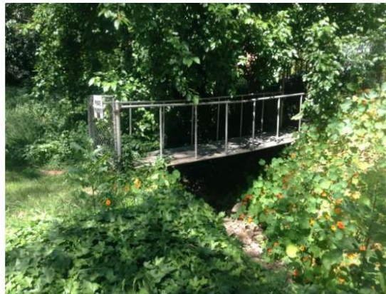
Defect – Overgrown Vegetation
