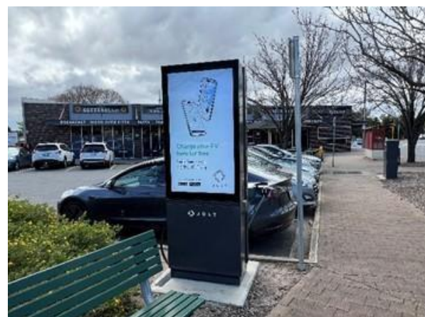
Jolt EV charging station in a private car parking on Newton Road
