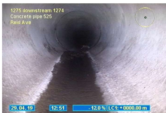
Typical underground SW pipe
