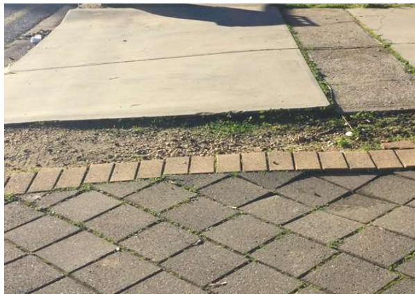
Missing sections of footpath
