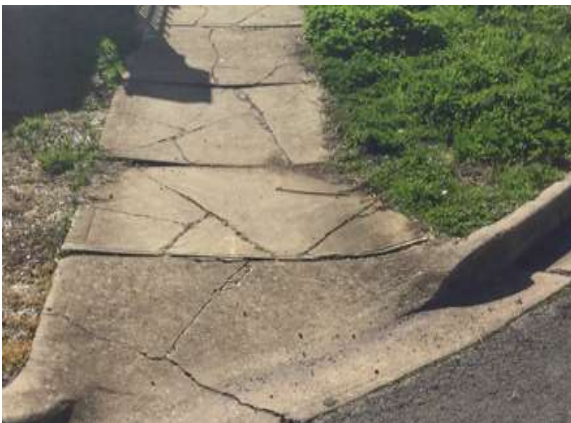
Cracking due to age and soil movements
