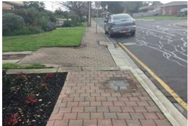
Depression caused water ponding
