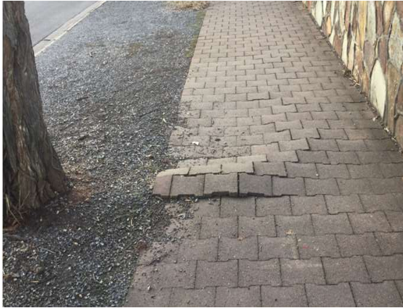
Tree roots causing paver lifts
